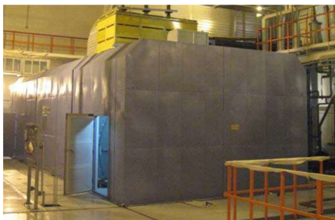
Fig. 3. Asynchronous condenser rated at 100 MVA.
